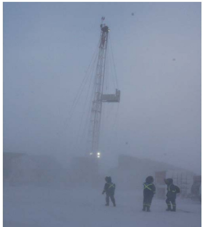
Nabors Service rig during storm. All personnel moving from camp to rig had to use buddy system. Winds slowed down rig up activities but work still advanced with caution.
